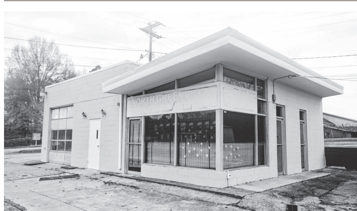
The building that formerly housed the North Greenville Food Crisis Ministry in Travelers Rest is being renovated.
